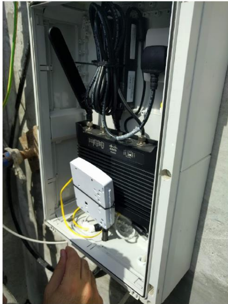
Cisco router in a cabinet
